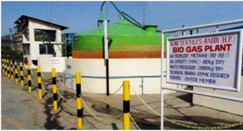
A Nisargruna biogas plant.
